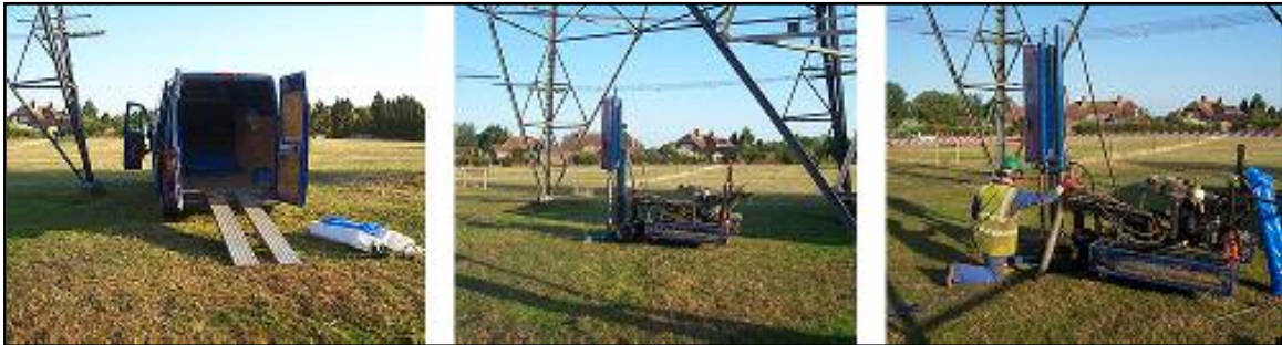
Figure 3: Window Sampler at work – Note the ability to be used even beneath a pylon.
